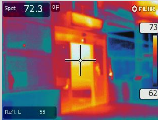
Infrared Heat Loss Image
